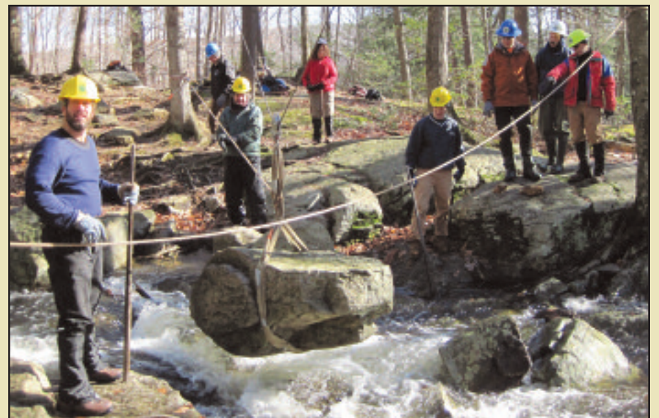
The Long Distance Trails Crew braved chilly, wet conditions to install new stepping stones.
