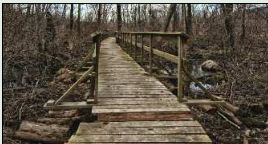
After one hard day's work by eight crew members, the bridge was ready for hikers.
