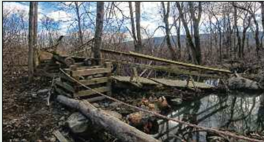
The Appalachian Trail bridge over Wawayanda Creek after flood damage last fall.
