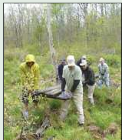
A crew of six man-handled the 500-pound, 16-foot long Beaver Brook Bridge back into place.
